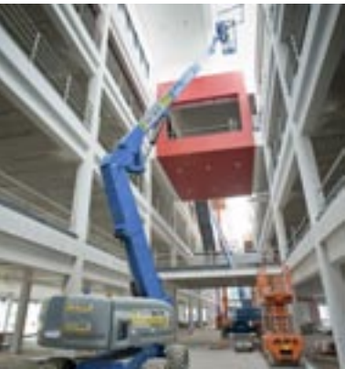
Safety platform access
